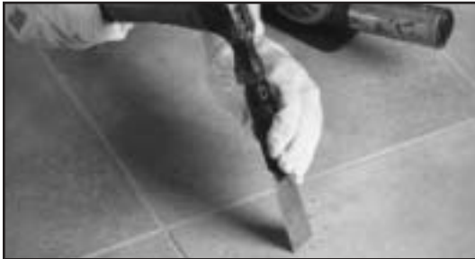
Fig. 19 - Drive a putty knife into the heated area and pry upward.
